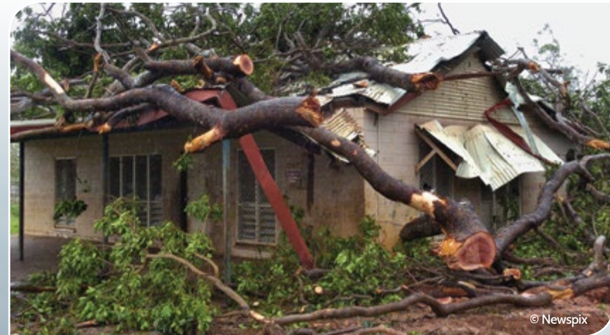
During Cyclone Monica in 2006, 75 per cent of houses in Maningrida suffered damage from strong winds or fallen tree branches.
