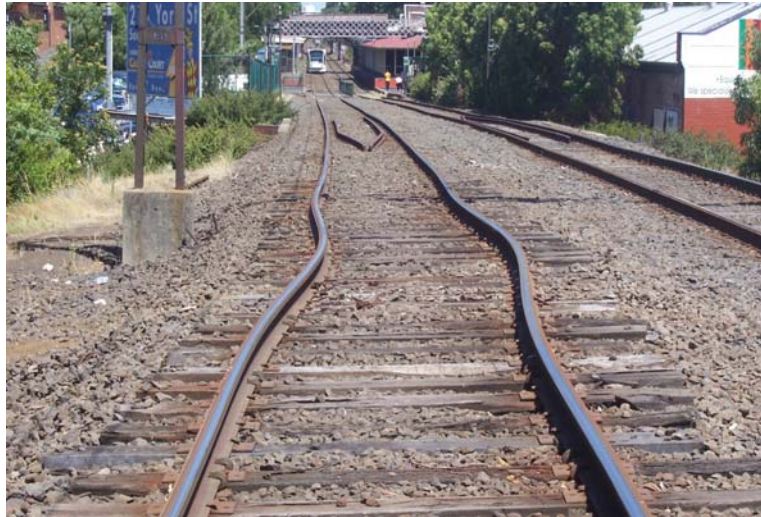
Figure 4.7 Buckled tram tracks due to the heatwave
