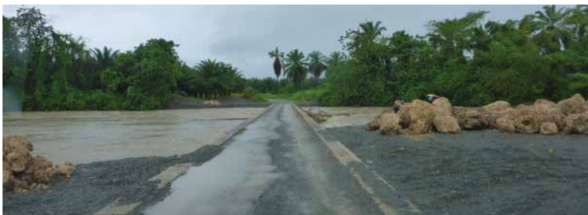
Figure 1: Flooding in Mberande
