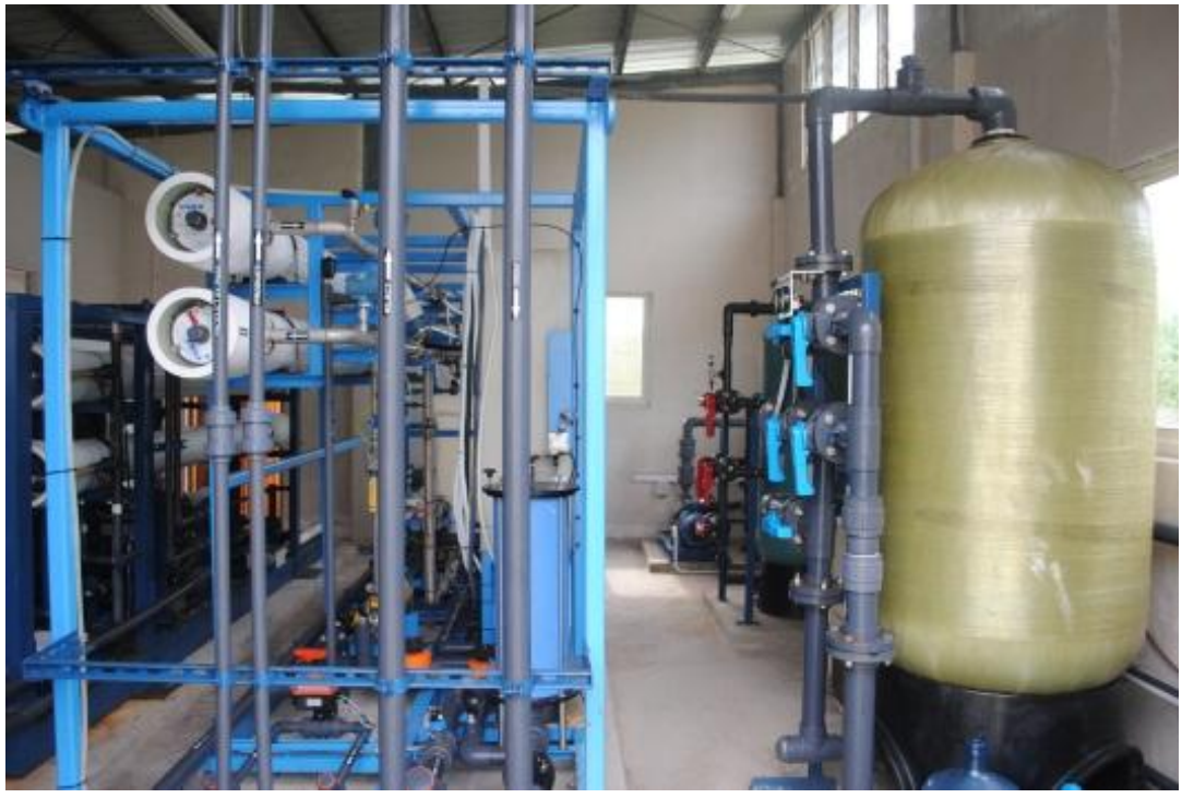
Figure 15: Desalination plant at the Public Works Department depot
